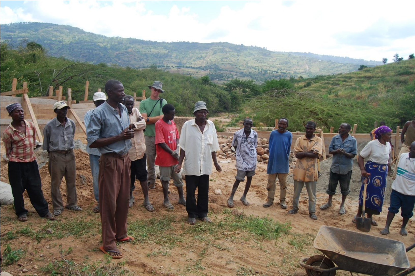
Sand dam building work party near Kola, Kenya. All photos: Dan Wiens
